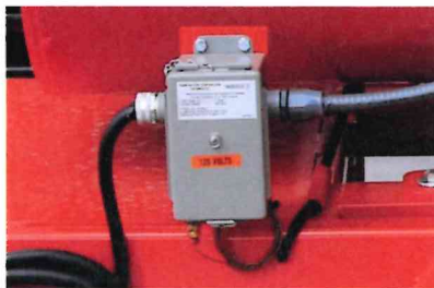
Overnight Heating System
