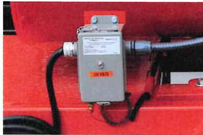
Overnight Heating System
