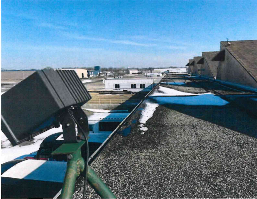
ALTERNATE 1 — Loose pea gravel will be leveled on the perimeter flat roofs.
