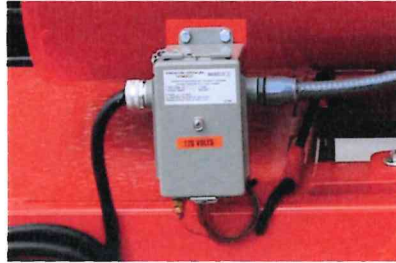
Overnight Heating System
